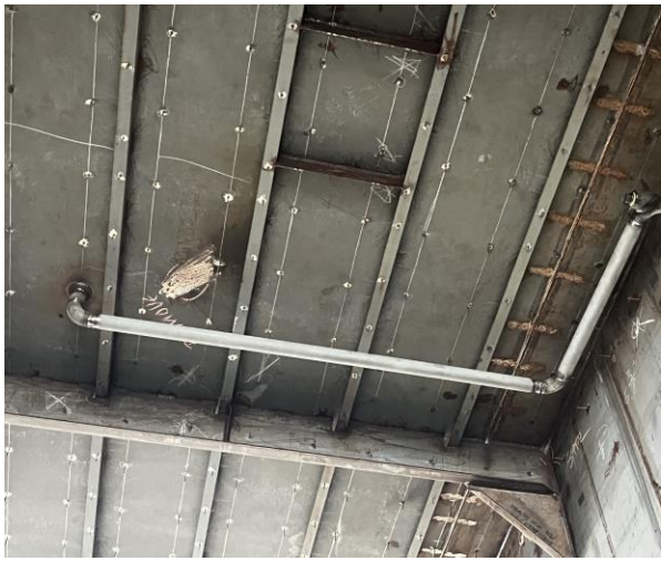
4136 – Piping and Insulation Studs in a 01 Deck Cabin
