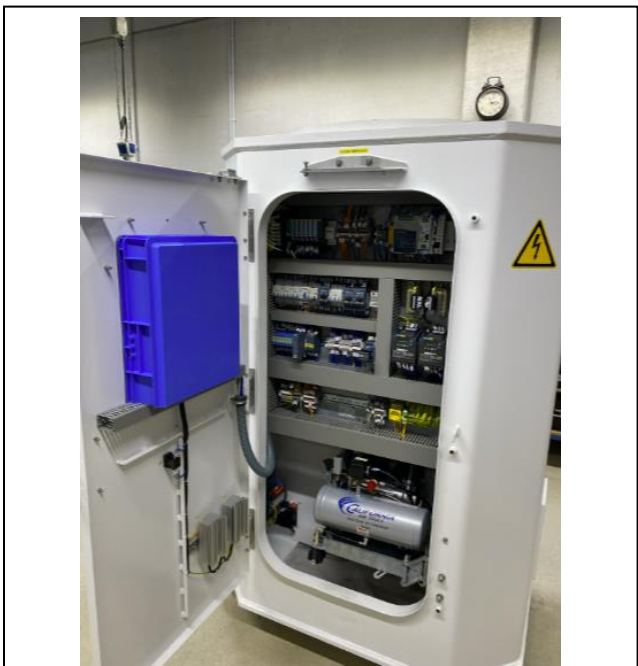
Charger 8 – Tower Base with Electrical Components
