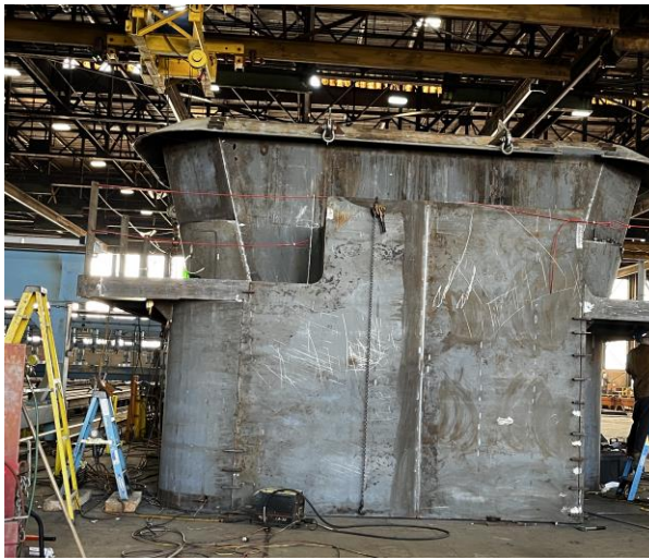
3957 – Pilot House on Deckhouse – Starboard Side (extended area of base is for elevator shaft)
