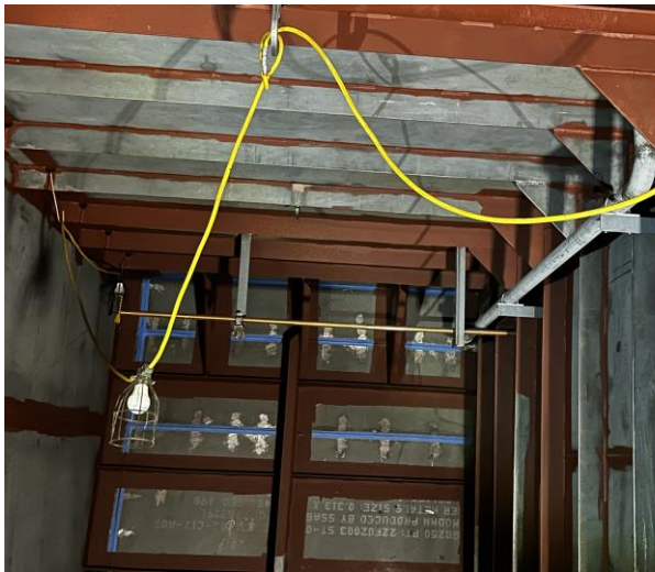
4011 – Partial Painting of Framing (red) and blue tape is to cover welds for a later inspection
