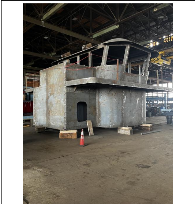
4124 – Pilot House on Deckhouse with Windows Cut Out – Starboard Side – Stern End
