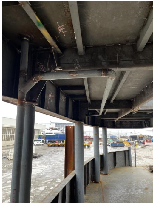
4012 – Deck Drain Piping on Starboard Stern
